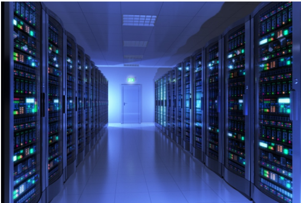
Data processing center
