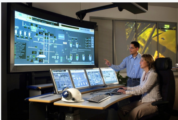
CCTV system protection
